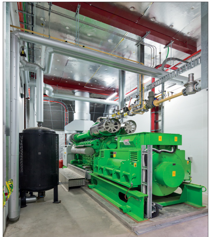
Figure 4 - Cogeneration engine within the Dandenong Energy Centre supplying electricity, heat and hot water within the Precinct
