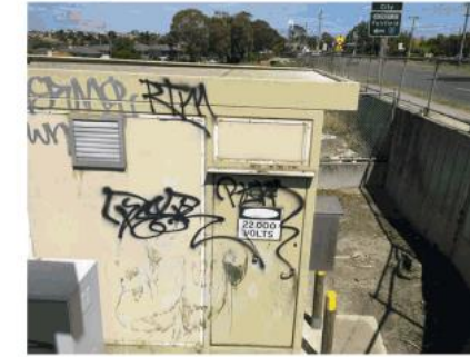
PLENTY ROAD VICROADS SUBSTATION
