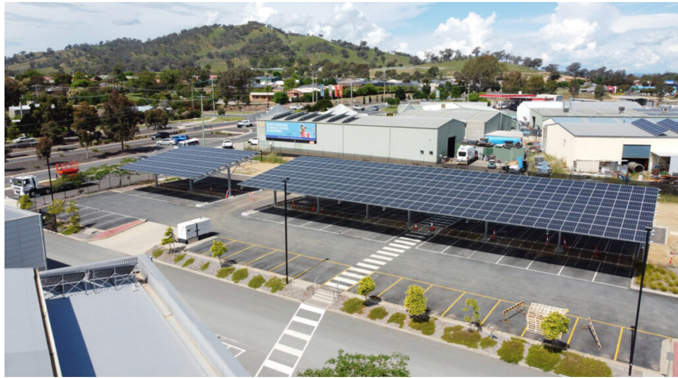
Carpark solar farm in Wodonga. Source: VicWater
