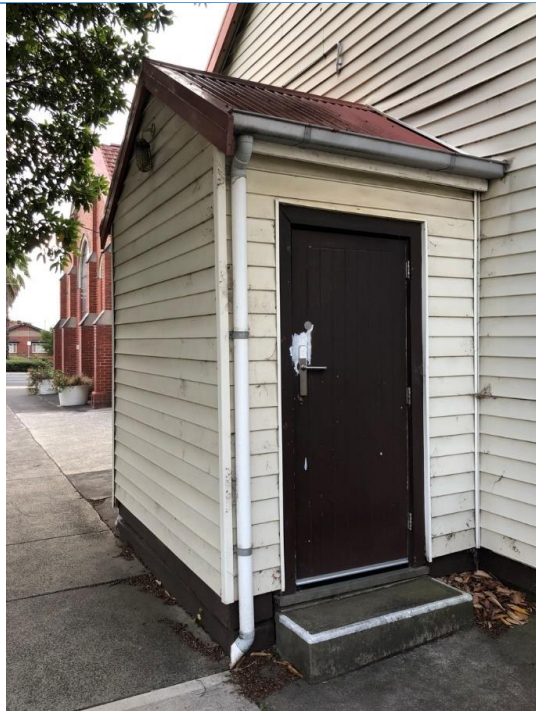
Northwestern view of the Church Hall, showing entrance. Source: Extent Heritage Pty Ltd, 2024.
