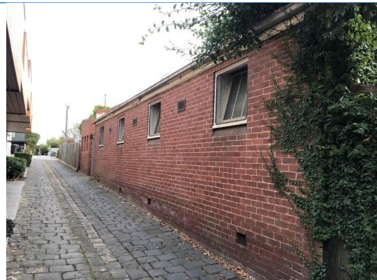
Oblique overview of the Kindergarten looking southwest. Source: Extent Heritage Pty Ltd, 2024.
