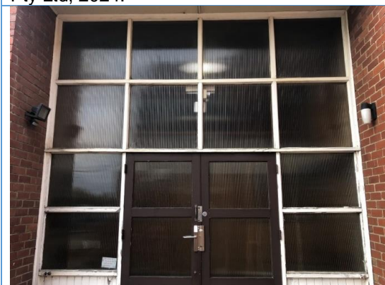
View of the Community Hall entrance glazing. Source: Extent Heritage Pty Ltd, 2024.
