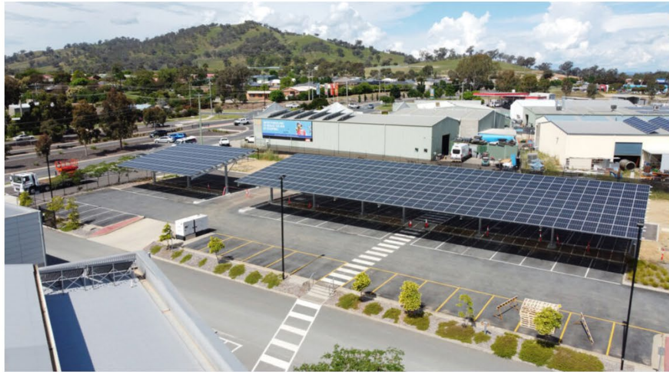
Carpark solar farm in Wodonga. Source: VicWater
