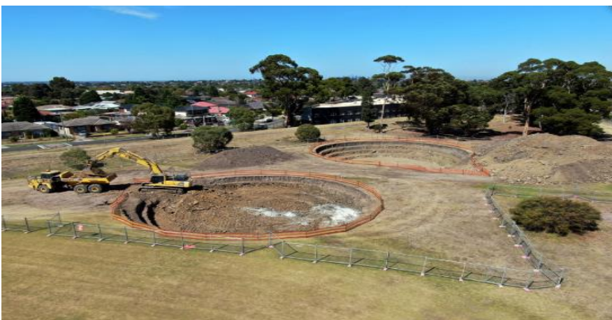
Figure 4: Making room for underground storage during construction of the harvesting system at Dole Reserve Reservoir.
