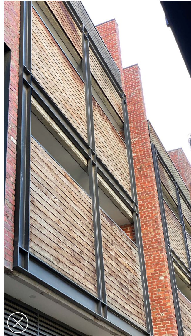
Privacy screens limit daylight and outlook from balconies and compromise amenities.
