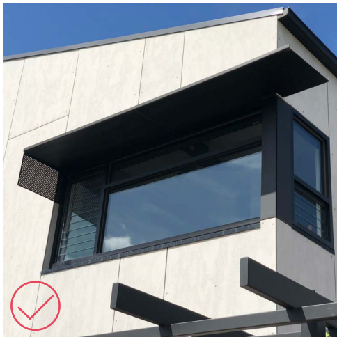
Large windows with hoods can allow for winter sun while restricting summer sun on the northern facade.
