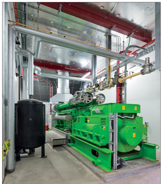
Figure 4 - Cogeneration engine within the Dandenong Energy Centre supplying electricity, heat and hot water within the Precinct
