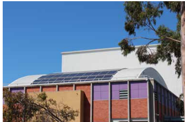
Solar panels on Darebin Arts and Entertainment Centre.
